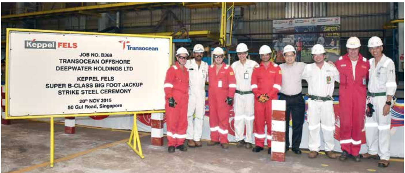
Cutting steel to mark the start of the construction of Project B368, a KFELS Super B Class design jackup rig, are project teams from Keppel FELS and Transocean
